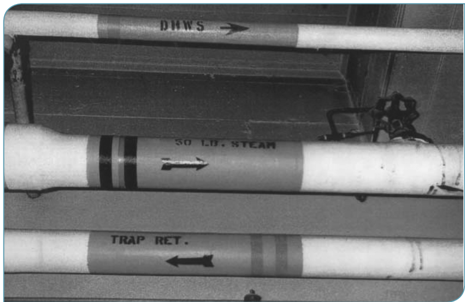
Hazardous products in pipes, identified by colours and letters
